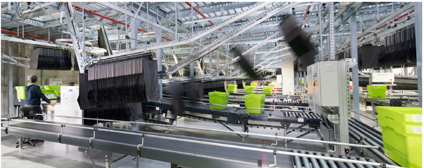
After induction to the Dematic Pouch System, the inventory flows on inclines up to the overhead dynamic buffer.
