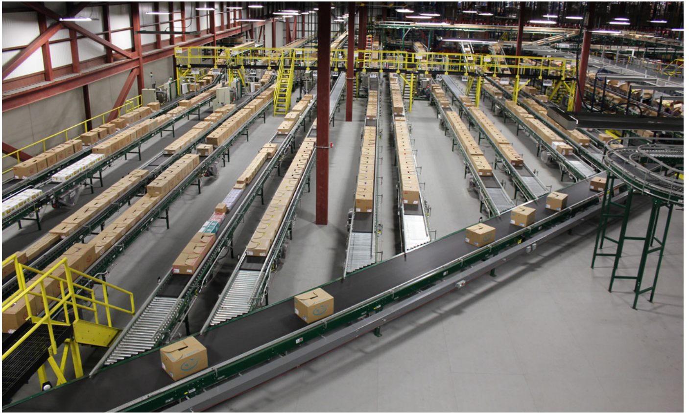
Cartons accumulate and merge prior to induction to the sorter.
