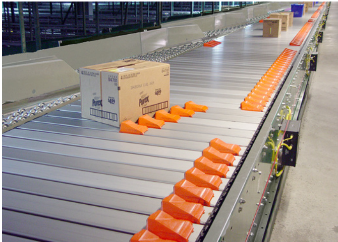
The Sliding Shoe Sorter diverts cases to shipping doors based on route, store, or carrier.
